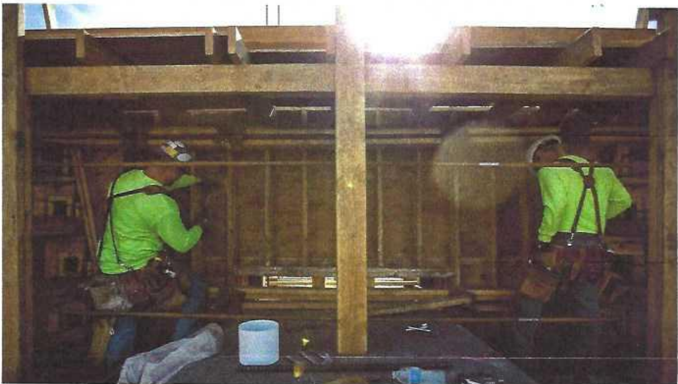
Carpenters in January work on a viaduct being built over Highway 99 in Fresno County as part of the California high-speed rail project. (Marcus Yam / Los Angeles Times)
